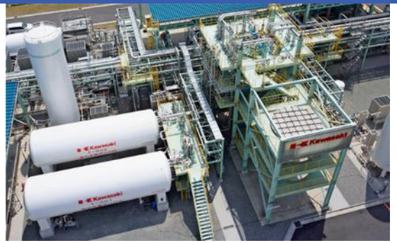
Hydrogen Liquefaction Plant
